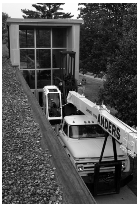
The crane was backed close to the north side of the Science Hall, providing the shortest reach to the tower.
